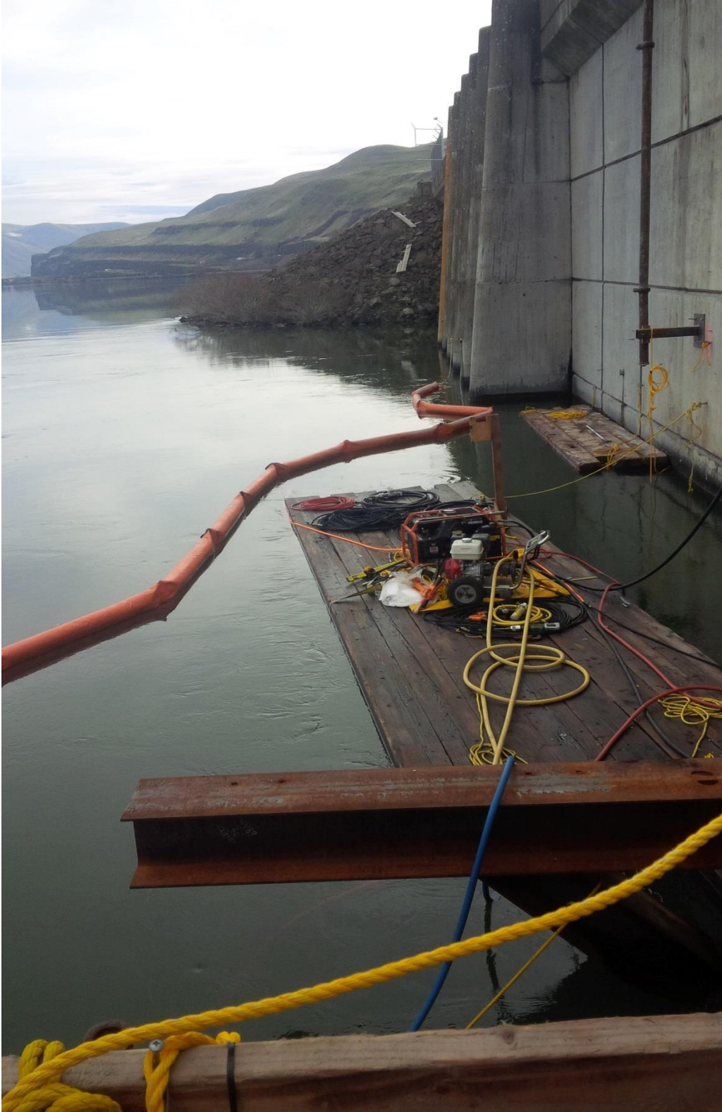
View towards east fishway exit from dive work platform. Requested boom gap correction.
