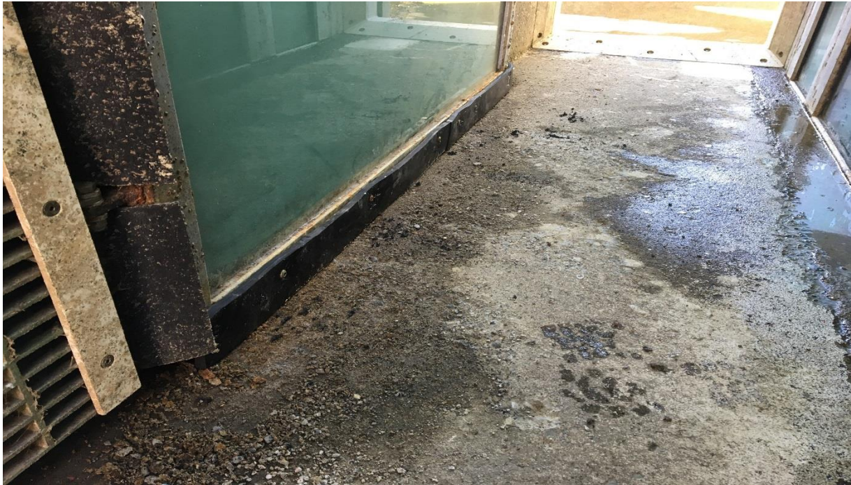
Rubber seal installed to prevent lamprey entry under east count station crowder.
