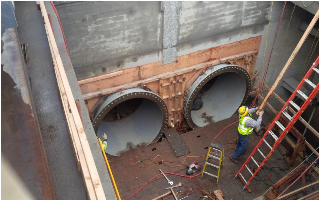
AWS 7' pipes entering AWS chamber west of junction pool
