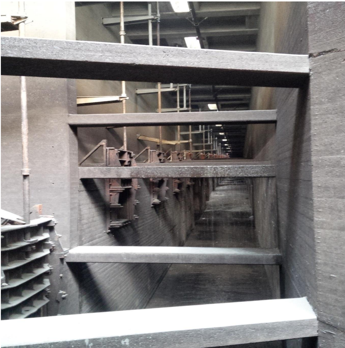
Failed support bracket for diffuser valve (slanted one). 4 others found with same failure.
