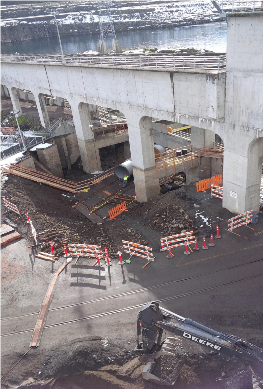
Installation of 7' pipe over junction pool. Could use more people pushing on it.
