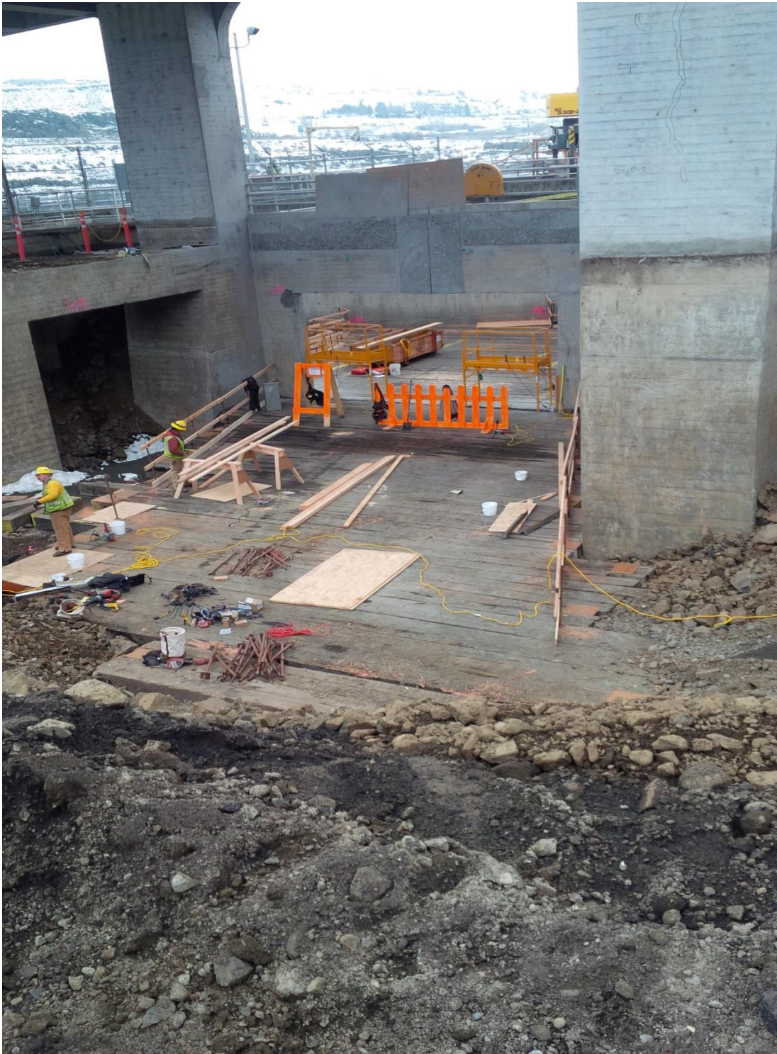
View from east face of junction pool. Opening for AWS pipe crossover.
