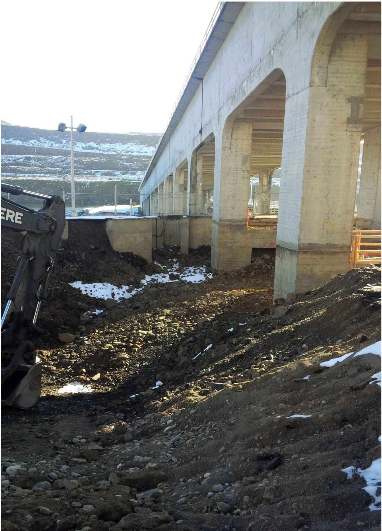
Excavation of valve place under east fishladder. Ready to cut junction pool wall.
