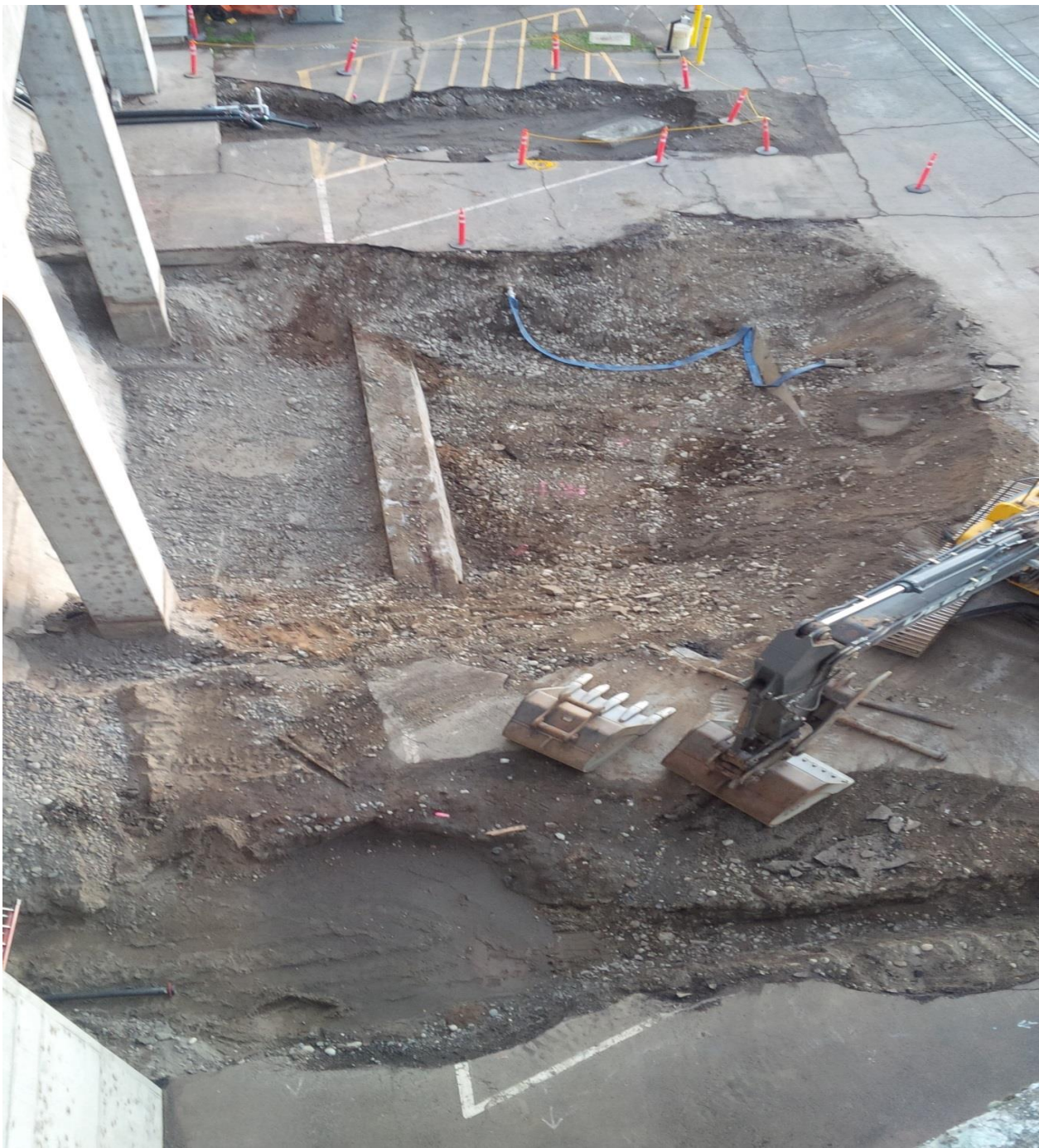
Unanticipated concrete beams discovered. Second beam barely visible under blue hose.
