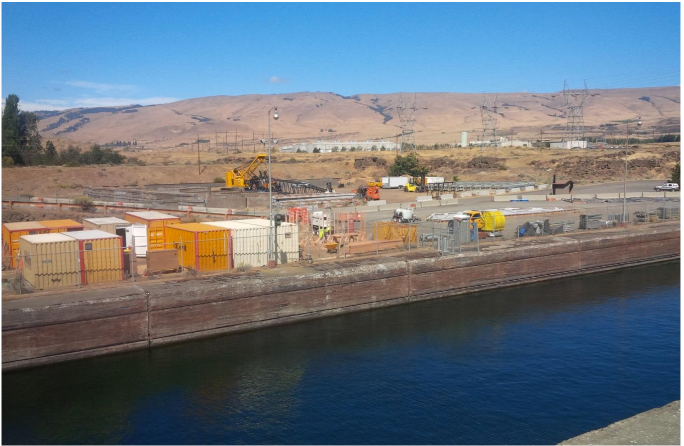
Mobilization and prefab work near navlock for start of EFL AWS construction this winter.
