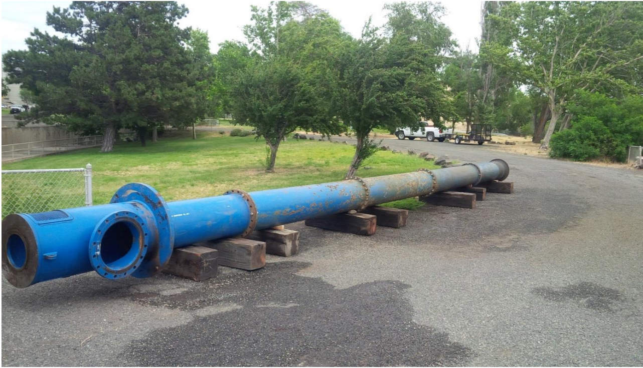
East fishway south dewatering pump removed for rehab. TO be completed for next winter.
