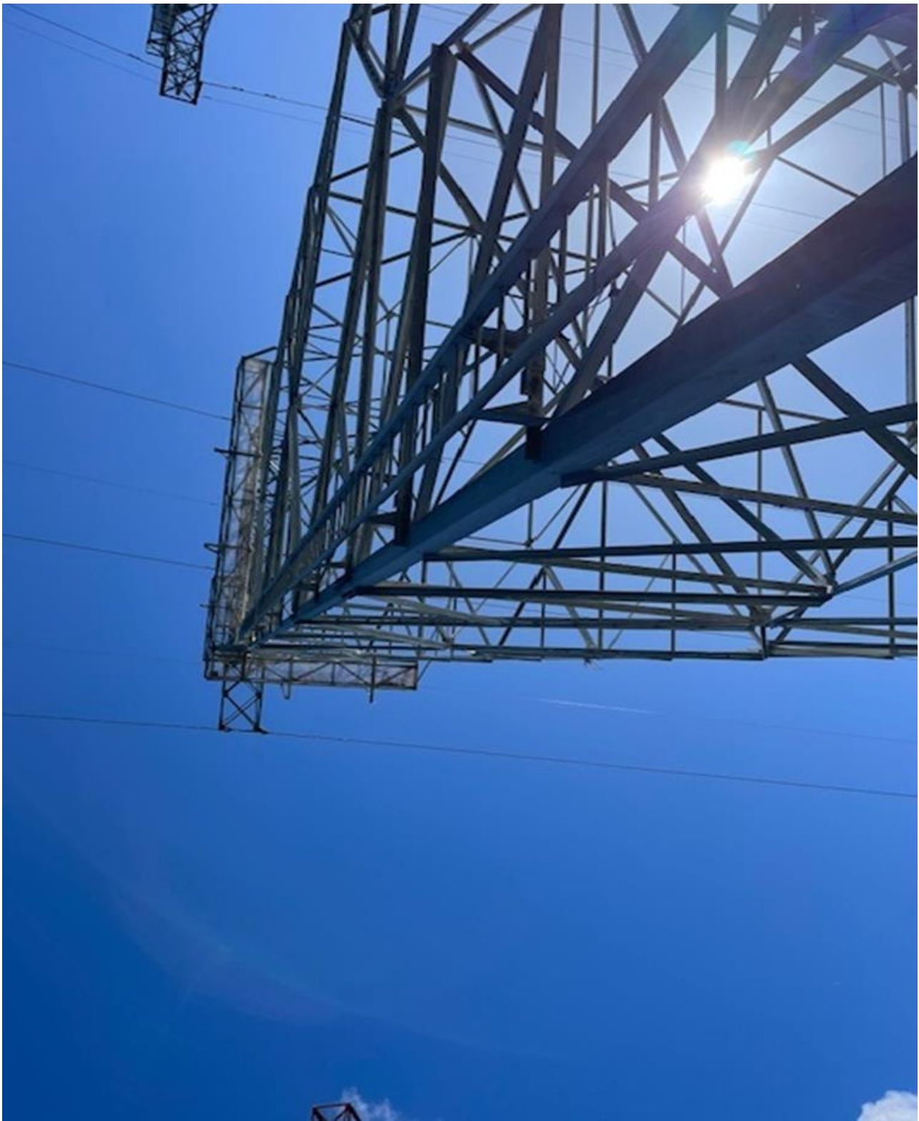
Middle tower walkway after nest removal on 3/14.. Speaker for Bird Gard is in corner of walkway.
