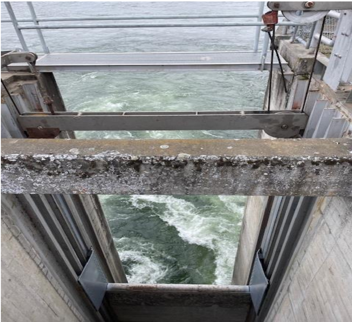
New Lamprey plates installed on weir E1. Remaining weirs planned for next winter outage.
