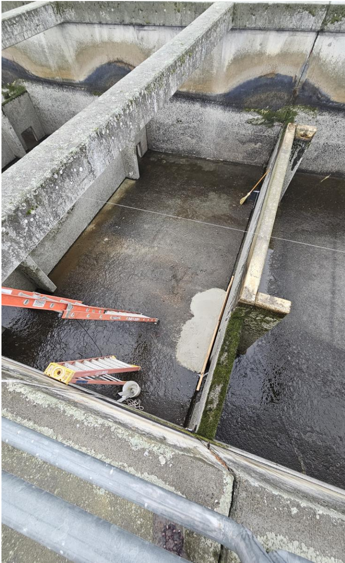
Expansion joint patchwork on the east fish ladder
