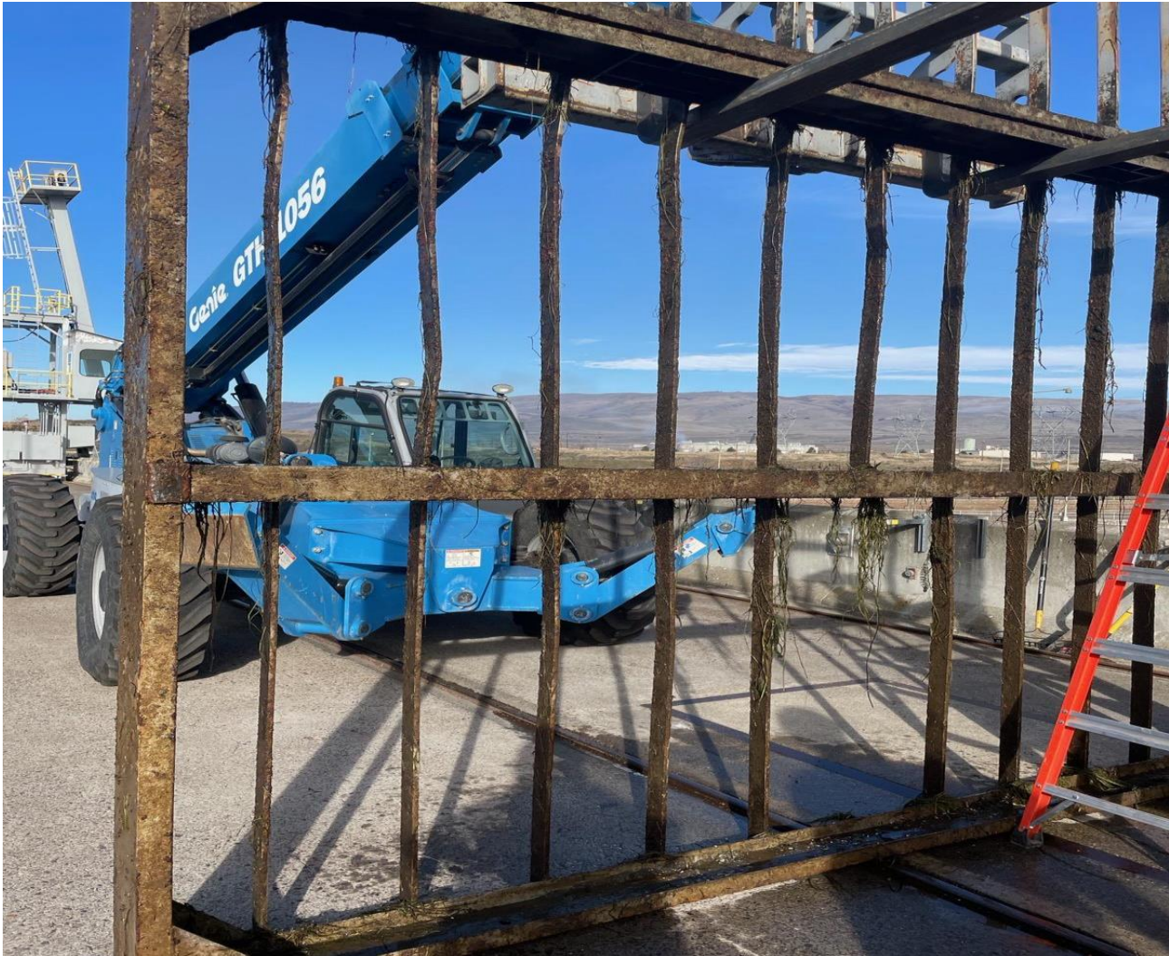
North ladder trashrack requiring minor repairs. Note bottom vane removed years ago for large strugeon egress
