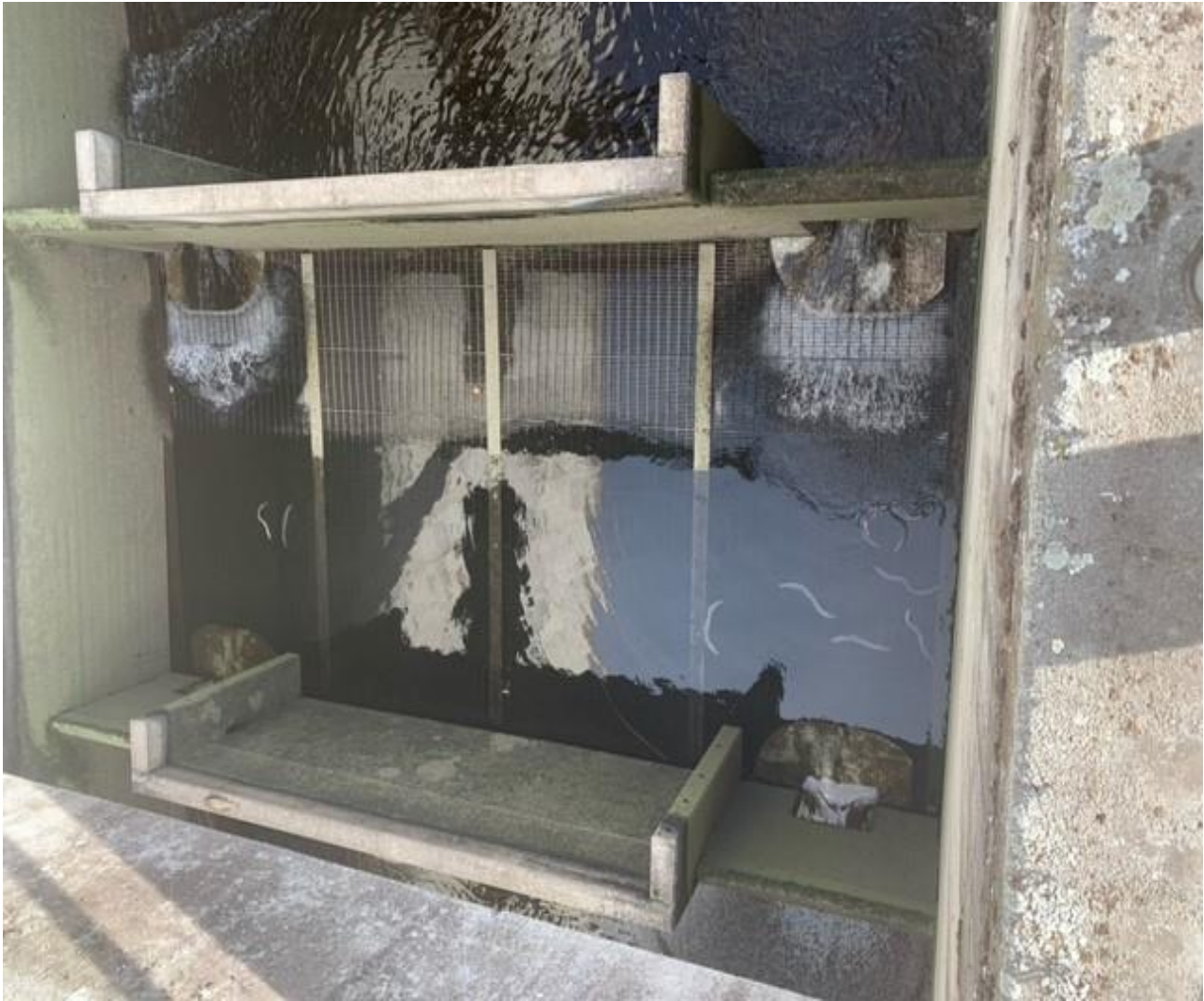
Lamprey mortality in east fishladder dewater. MFR provided to FPOM.
