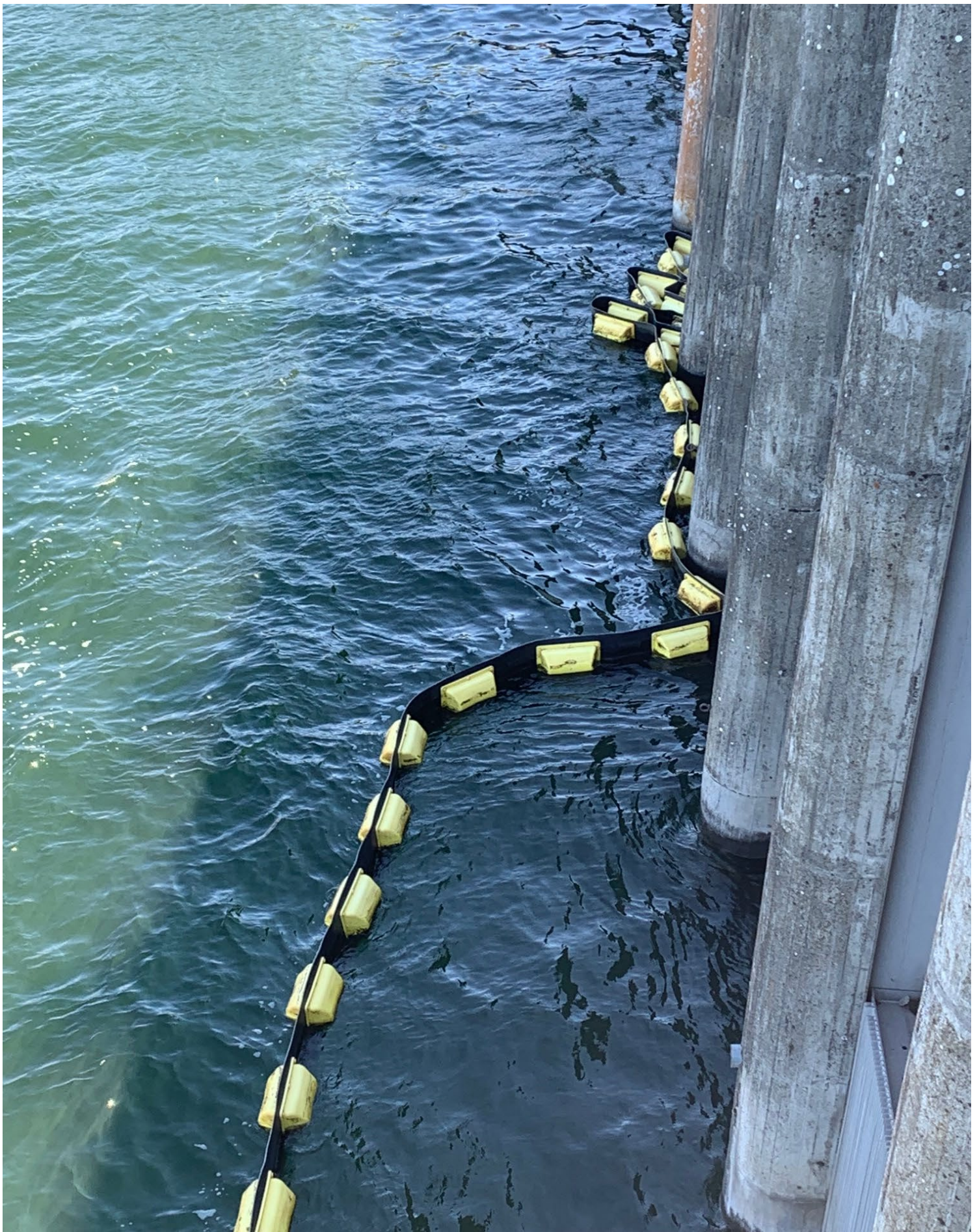
Boom at East Exit failed at upstream attachment
