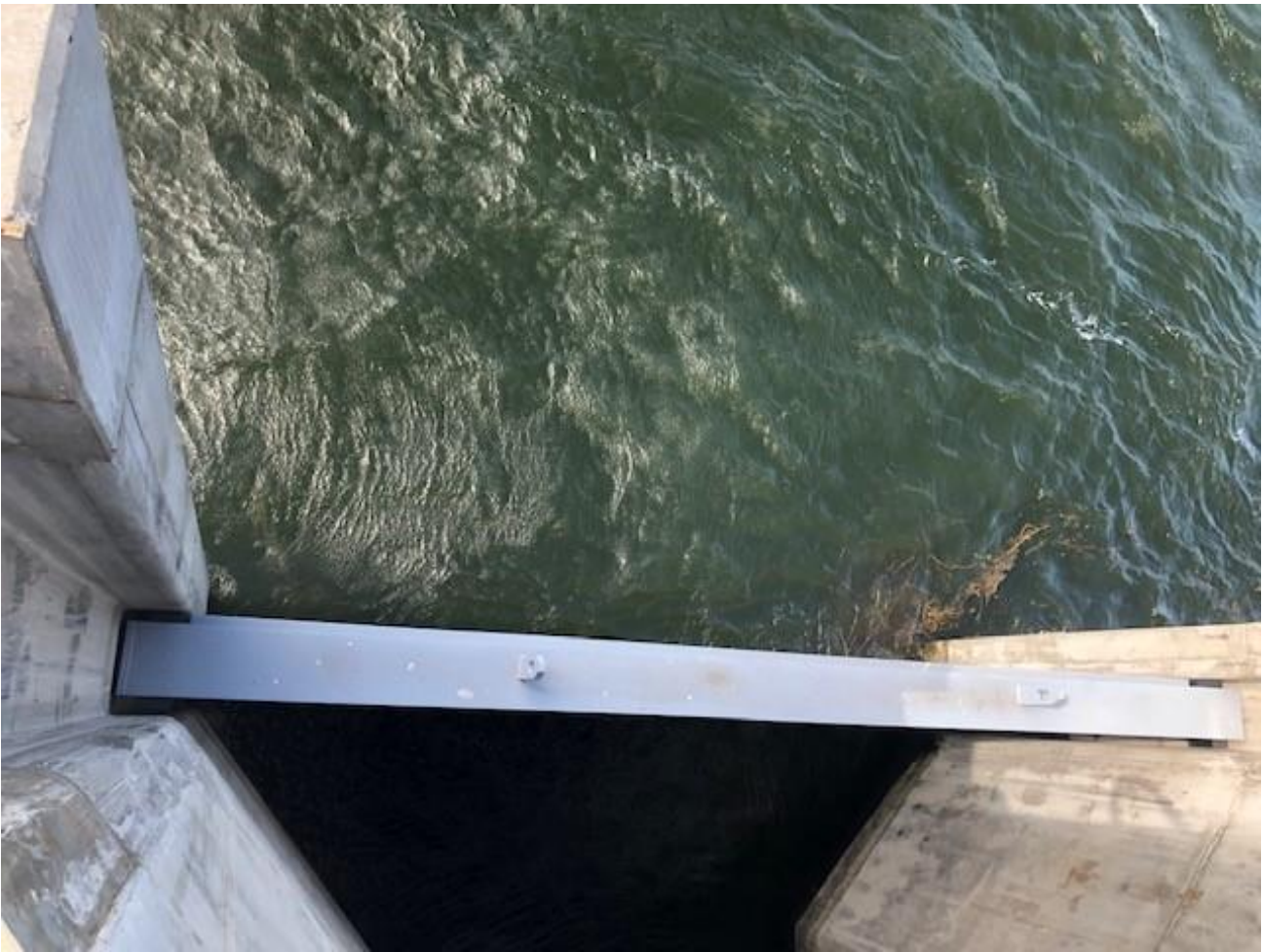
AWS intake, floating off debris during close cycle
