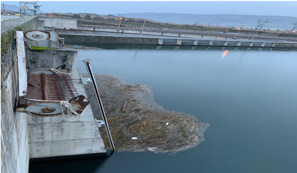
North PUD intake with high debris loading. Rake system out of commission.
