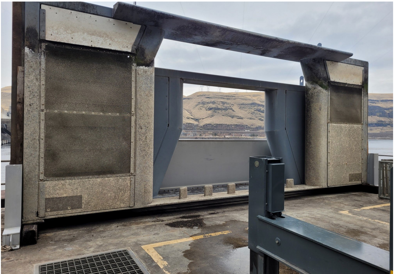
NFL Entrance Weir staged for downstream UHMW panel replacement. The image is of the downstream side. Currently there are STS mesh panels in lieu of UHMW panels. This is the lowest panel when deployed. The other 2-panels are stacked visibly behind.
