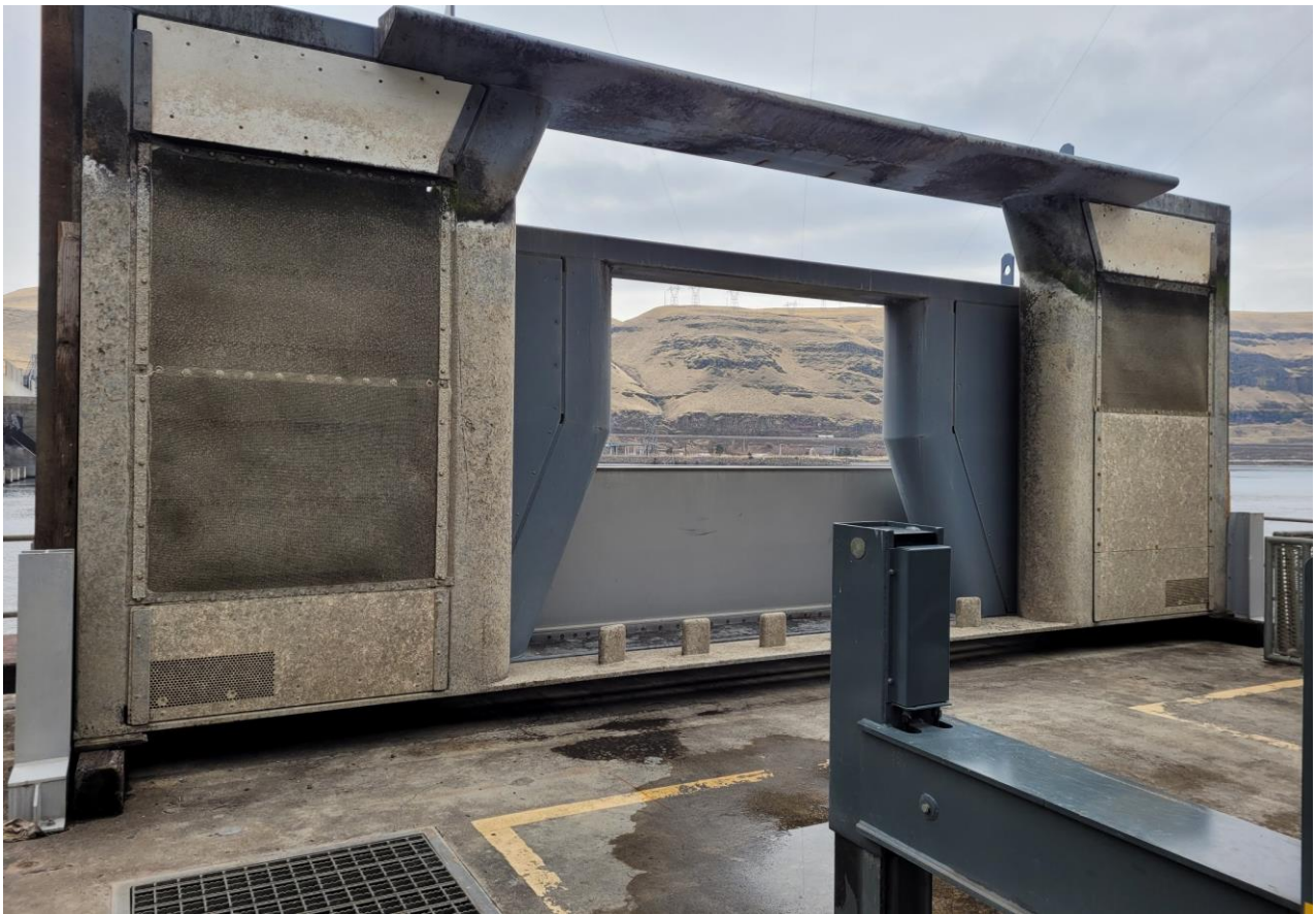
NFL Entrance Weir staged for downstream UHMW panel replacement. The image is of the downstream side. Currently there are STS mesh panels in lieu of UHMW panels. This is the lowest panel when deployed. The other 2-panels are stacked visibly behind.
