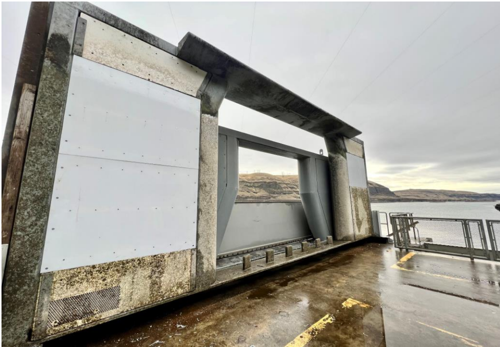
NFL variable width entrance weir with UHMW panels installed.
