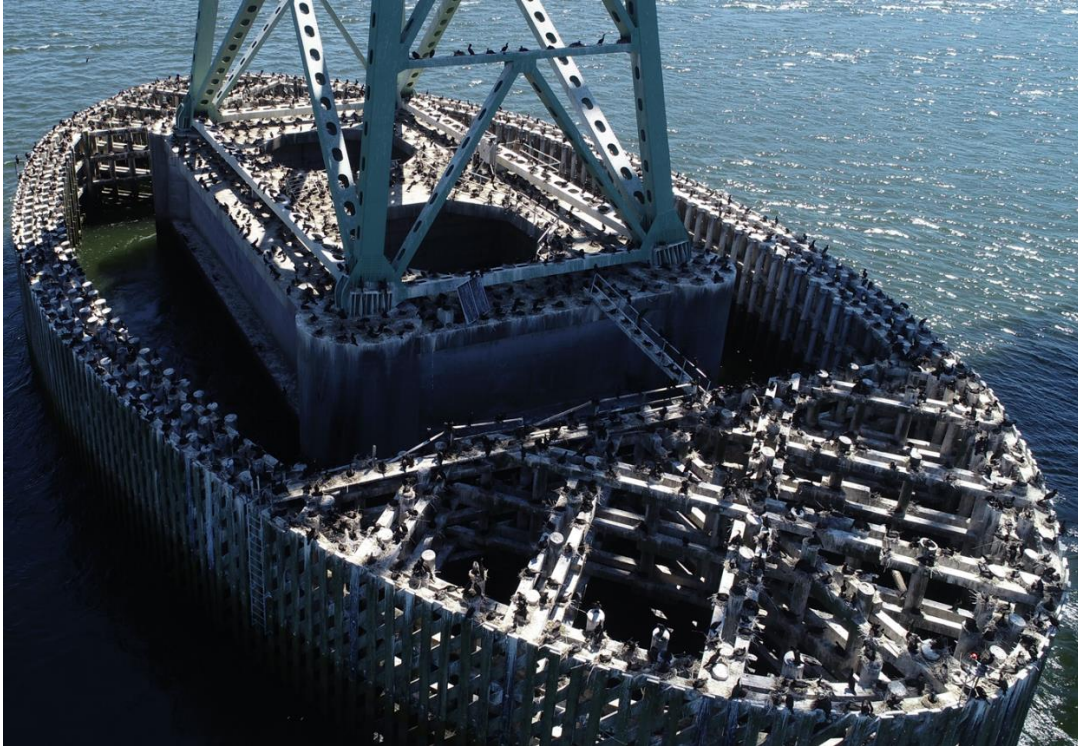
Figure 4. Double-crested and Brandt's cormorants nesting on the north crib of the Astoria-Megler Bridge from a RTR June 2, 2021 drone survey.
