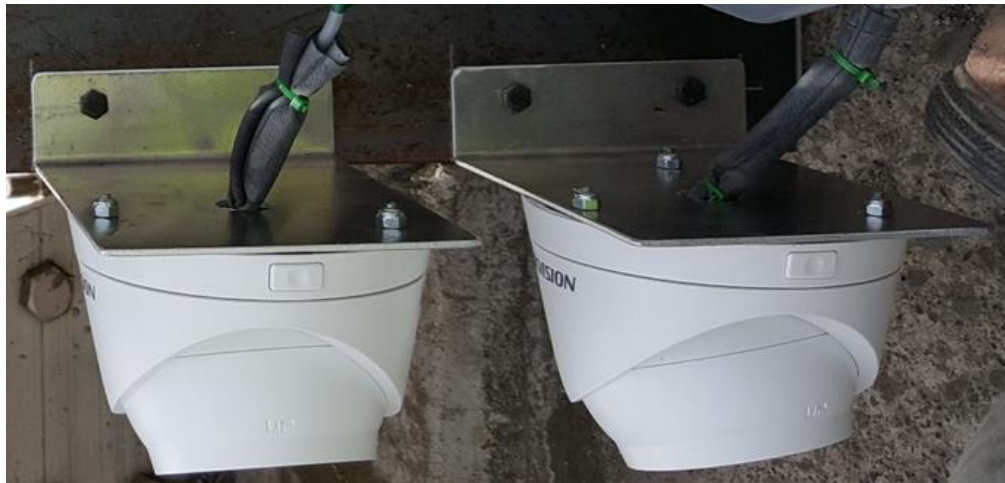
Figure 17 Photograph of Video Cameras Mounted on Steel Brackets
