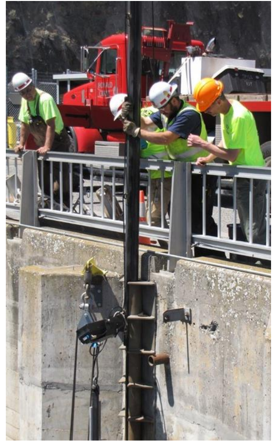
Figure 4 Photograph Showing Deployment of the ARIS/rotator Assembly Through the Trolley Pipe Adjacent to the North Edge of the Fishway Exit
