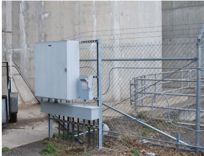
Figure 8: Electrical Equipment near Fishlock
