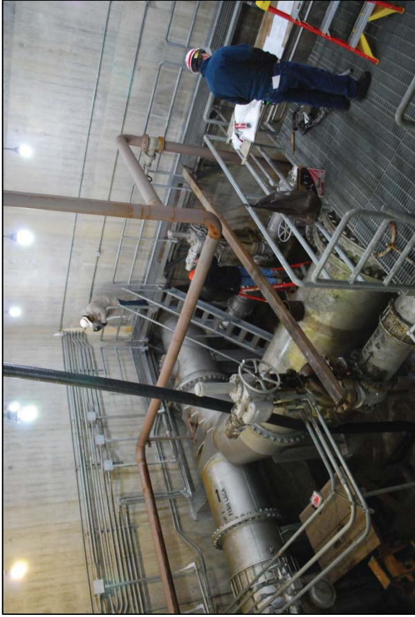
Photograph 1 . Typical View in Valve Room .
