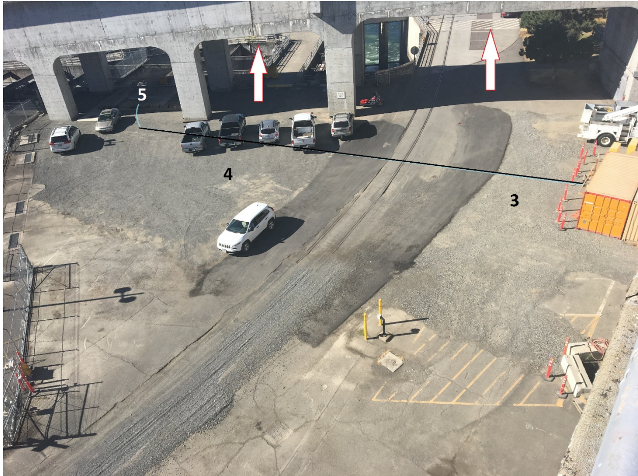
Figure 1.1. Construction Site at The Dalles Dam Fish Ladder. The excavation area is marked with the black line numbered from 3 to 5.
