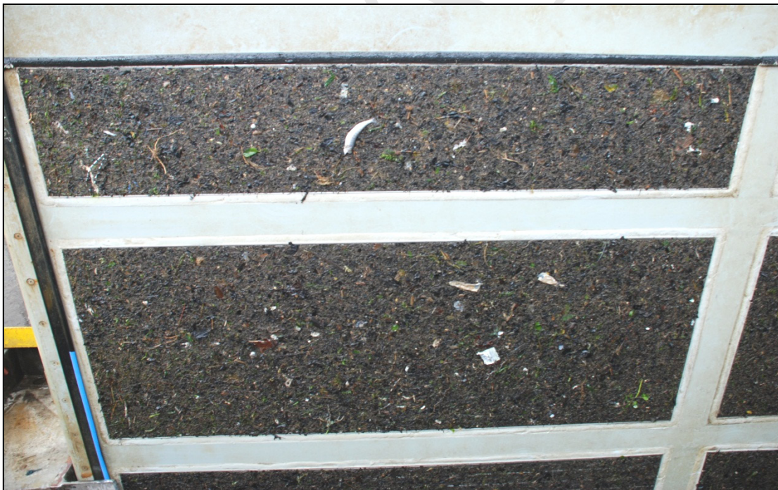
Figure 9. Bonneville Dam Second Powerhouse VBS panel on 19 May 2008. Photo shows the lower VBS section clogged with debris.
