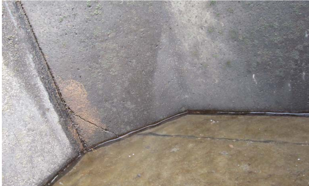
Figure B2.4.22 Crack in Channel Leading Up to Exit
