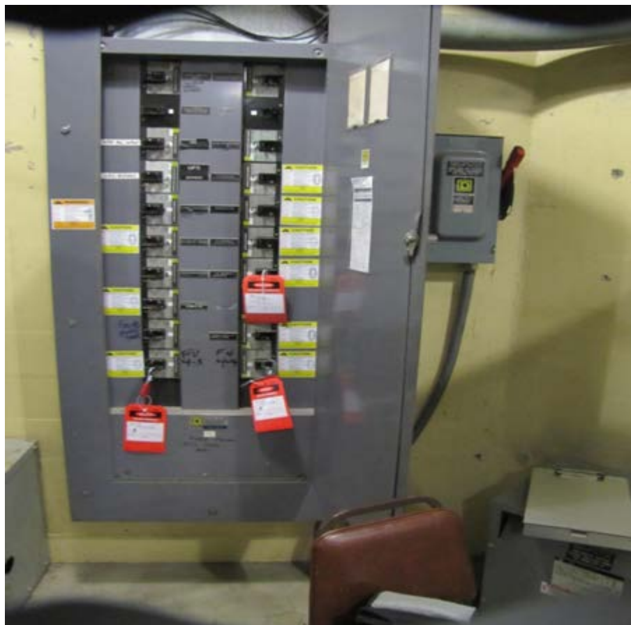
Figure B1.6.14 Panelboard FP-3. (Note tag-out tags for gate operator power.)
