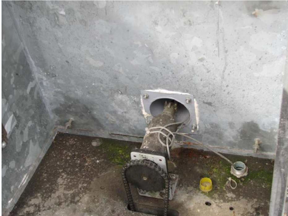
Figure B1.6.5 Duopot Position Transmitter for Intake Gate
