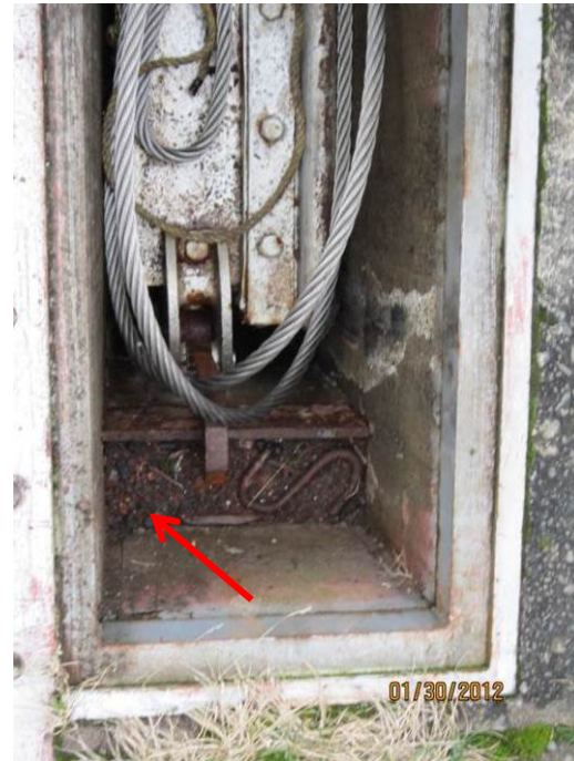
Figure B2.4.29 Corrosion around Bulkhead.
