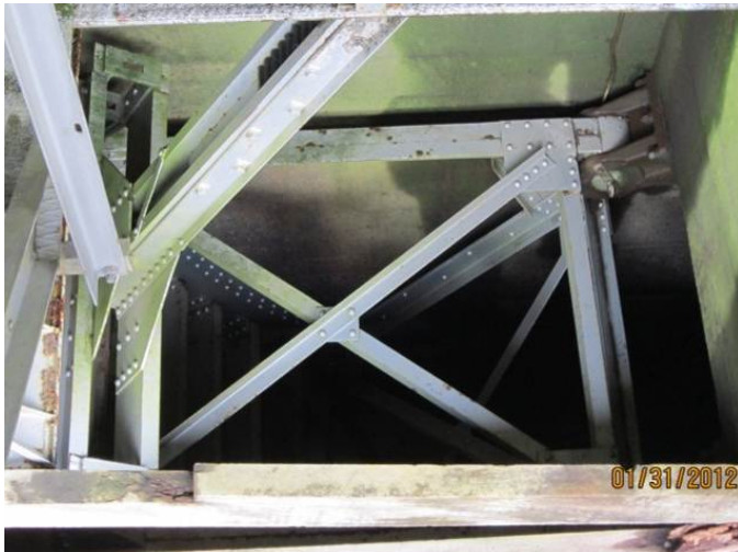
Figure B2.4.35 FV3-8, Mechanical Components
