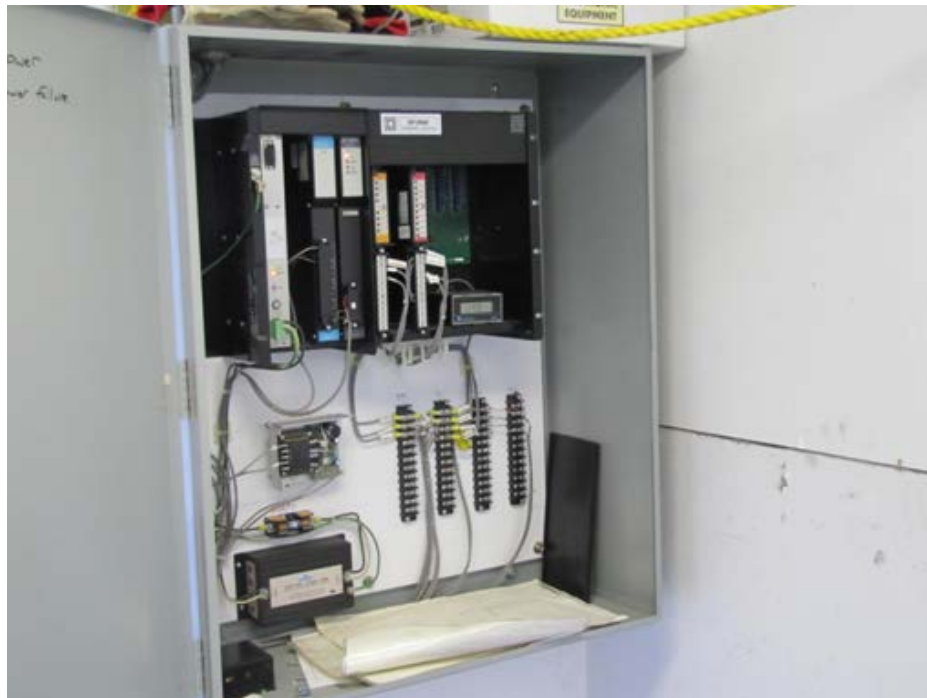
Figure B1.6.8 Enclosure with Remote I/O Rack
