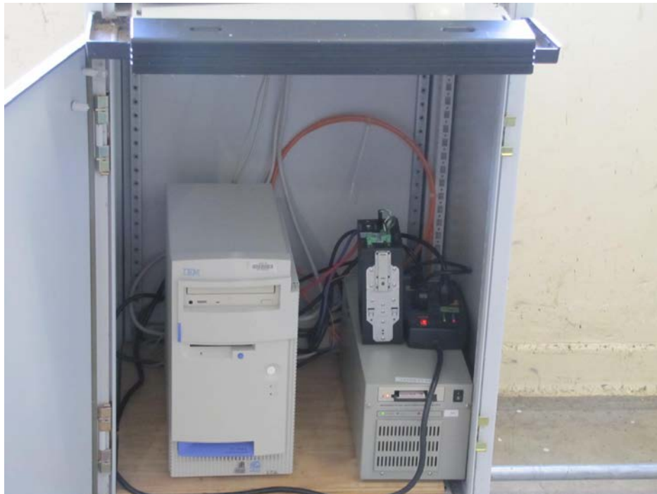
Figure B1.6.9 Soft PLC Located in the Power House Control Room for Operation of the Fish Ladders
