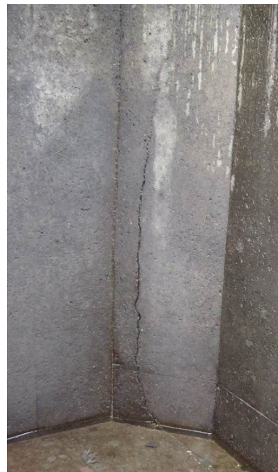
Figure B2.4.21 Crack in Channel Leading Up to Exit
