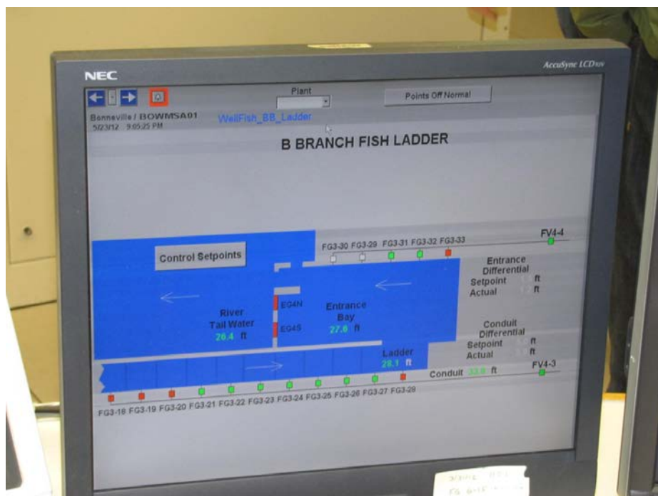
Figure B1.6.12 HMI used for B Branch Fish Ladder Operation
