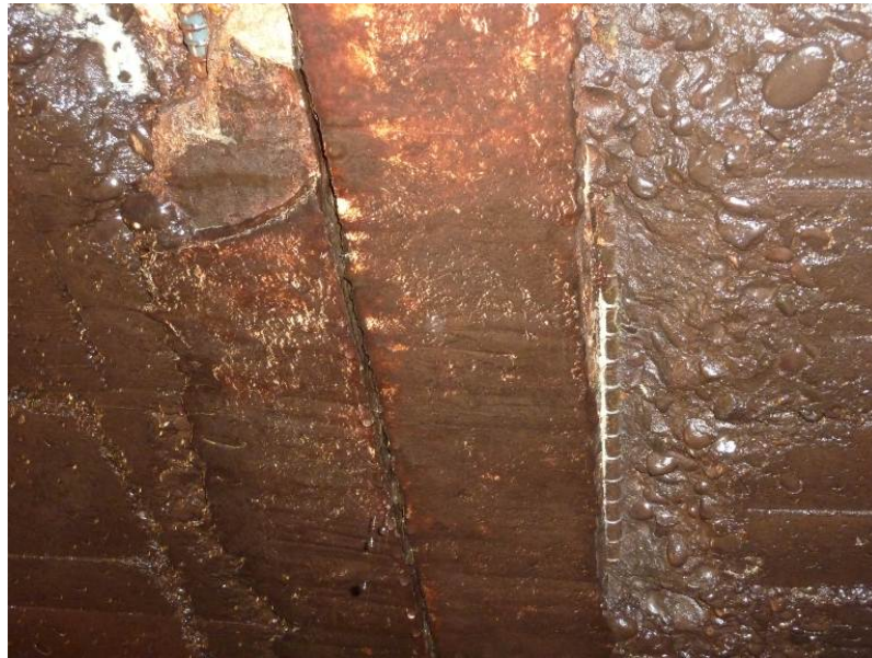
Figure B2.4.19 Joint with Exposed Rebar and Waterstop along Ceiling
