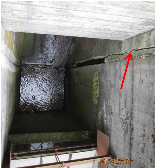
Figure B2.4.8 Cracks in Walls of Fish Lock Structure
