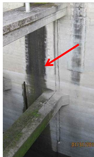
Figure B2.4.13 Crack in Wall
