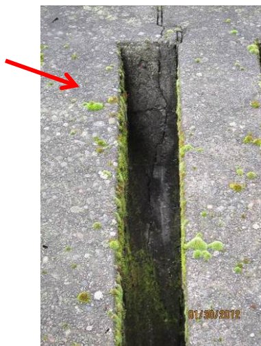
Figure B2.4.12 Crack between Expansion Joints at Weir 43
