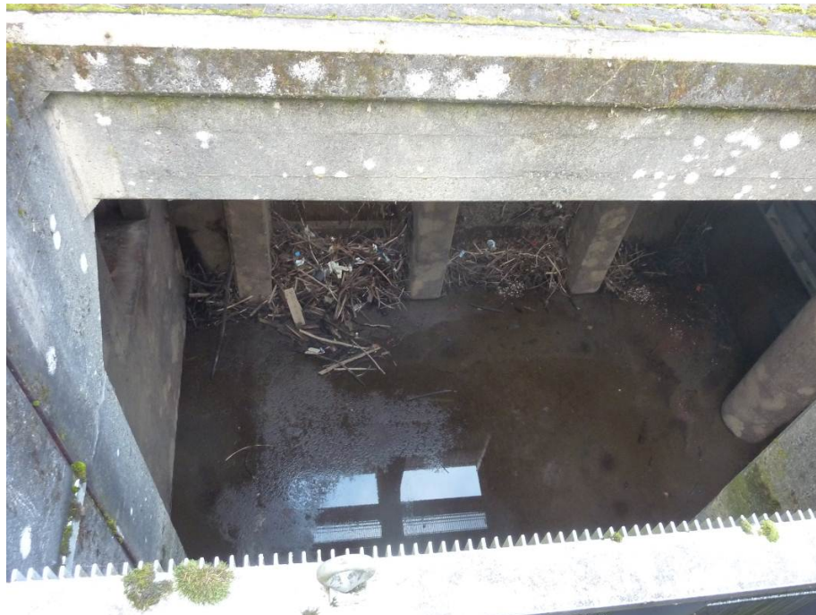
Figure B3.4.12 Equalization Chamber viewed from above.
