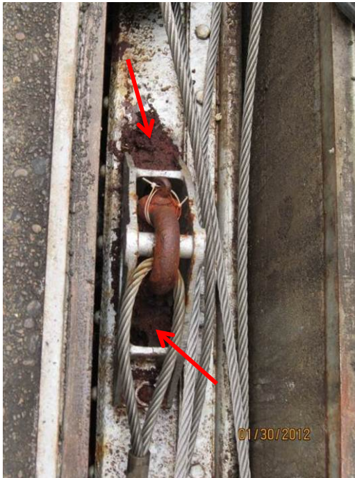
Figure B2.4.28 Corrosion around Bulkhead.
