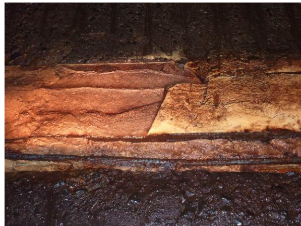
Figure B2.4.18 Joint with Exposed Rebar and Waterstop along Ceiling
