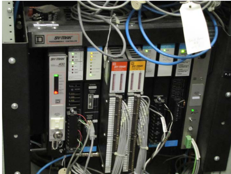
Figure B1.6.13 Remote I/O rack for communication with PLC
