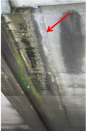
Figure B2.4.4 Cracks in Walls of Diffuser Structure
