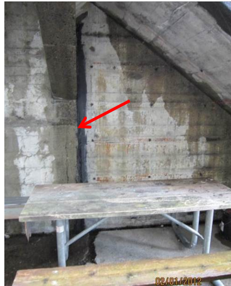
Figure B2.4.9 Cracks in Walls of Fingerling Bypass Structure
