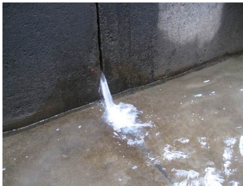
Figure B2.4.24 Leak in the Waterstop
