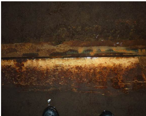
Figure B2.4.17 Joint with Exposed Rebar and Waterstop along Floor
