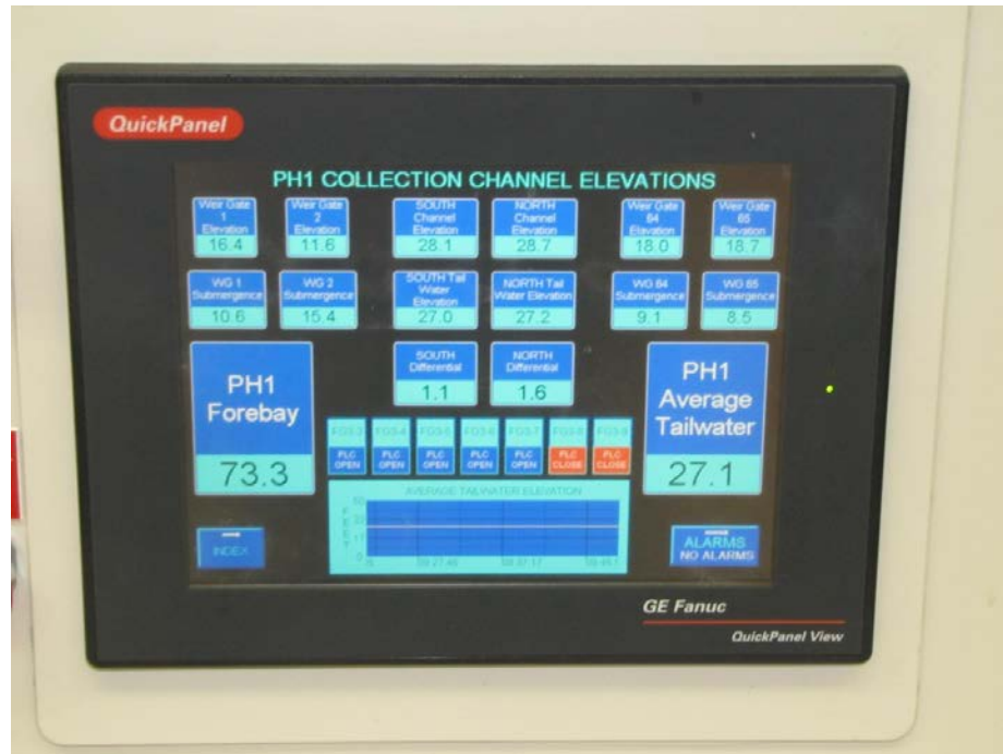
Figure B1.6.10 HMI Located in Power House Control Room for Operation of the Fish Ladders
