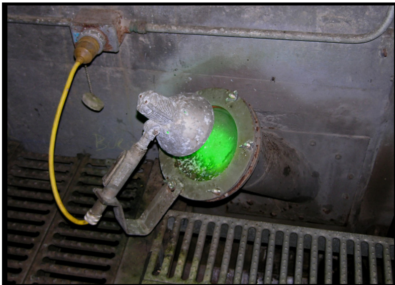
Figure 2.3. Light-emitting diode light installed above light tube at Orifice 12A South
