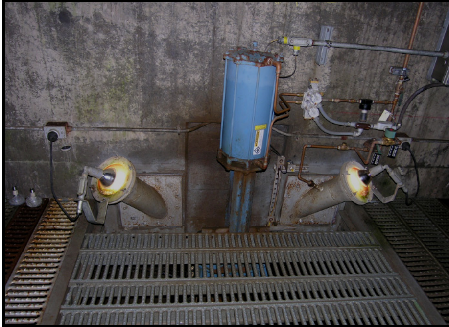
Figure 2.7. Top portion of light tubes in downstream migration channel with halogen lights installed
